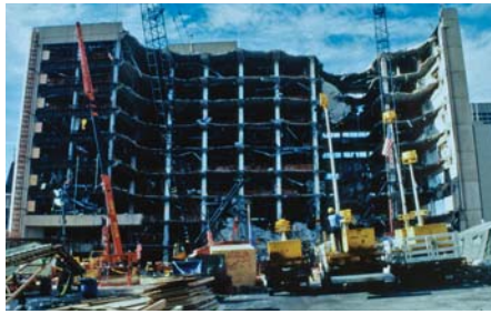
The Alfred P. Murrah Federal Building in Oklahoma City, one week after it was destroyed in a right-wing terrorist bombing on April 19, 1995.
